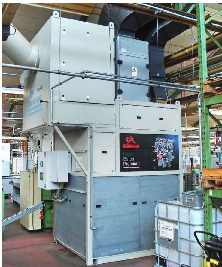
Heat recovery systems reduce gas consumption.
